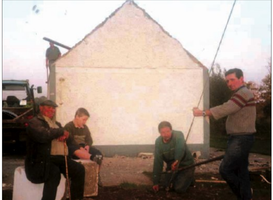
The demolition of the old dressing rooms in October: "Clerk of works" Neddy Aldridge keeps an eye on John Joe Aylward and Anthony Conway
