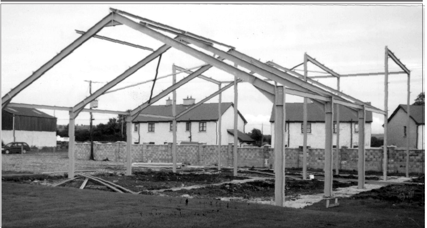
The steel frame of Cloneen's new Clubhouse and Handball Court, under construction Oct. 2000
