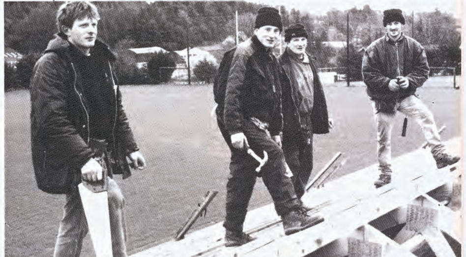
RAISING THE ROOF IN WINDGAP - Carpenters at work on the roof of the new dressing rooms in Windgap, l-r: Gay Doyle, John McKenna, Paddy Walsh (contractor), Ray Dunne.
